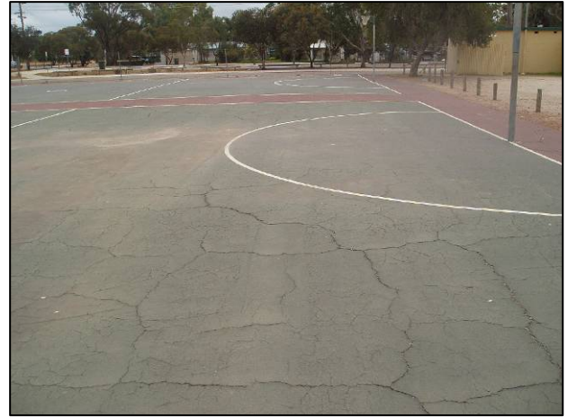
Heavily cracked surface
