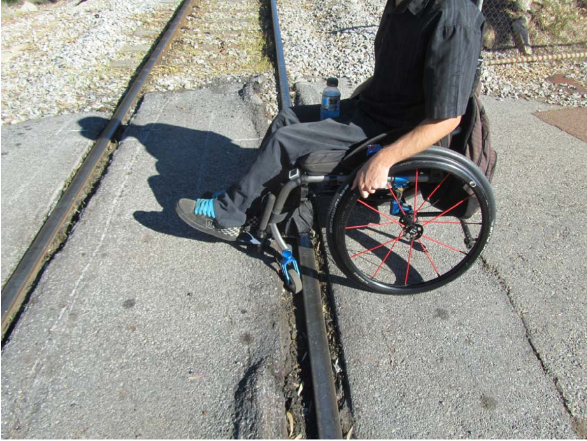
Macartney Street railway crossing so bad that wheelchairs get stuck in the lines and gophers drive across the line in the middle of the road as the sides are so uneven. (since these photos were taken Brookfield Rail has re bitumised this section)
